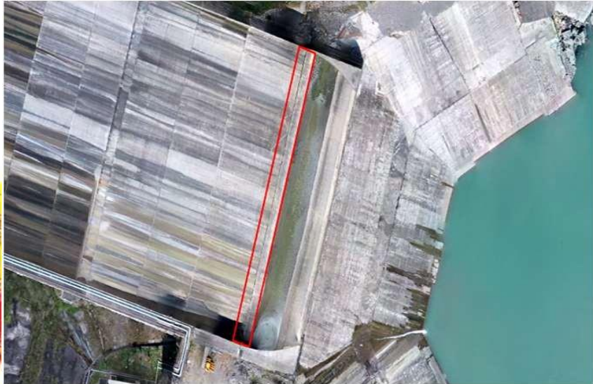
Crack / Spillway Analysis
